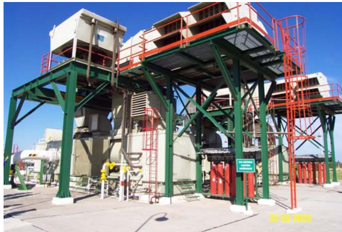
Figure 4 – Weather Exposed Compressor Station in Argentina
